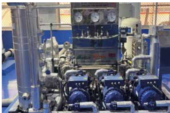
Figure 1: R744 Chiller for ship cooling application, Q_o=100 kW, Chilled water 12^{\circ}\text{C} to 7^{\circ}\text{C} , seawater temperatures up to 36^{\circ}\text{C} .
