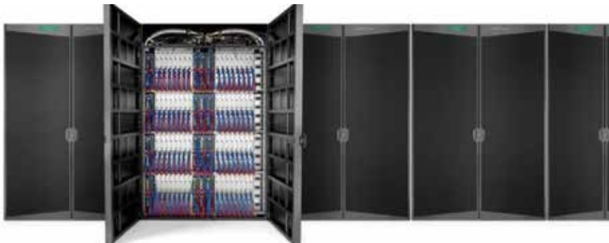
Figure 5: High-Density Liquid-Cooled Server Rack Infrastructure.
