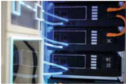
Figure 3: Direct Liquid-Cooled Hardware in a Modern Data Centre.
